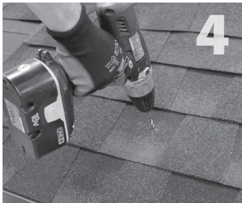
4 Using drill with 7/32" bit, drill pilot hole into roof and rafter, taking care to drill square to the roof. Do not use mount as a drill guide. Drill should be 'long style bit', aka 'aircraft extension bit' to drill a 1 3/4" deep hole into rafter.
