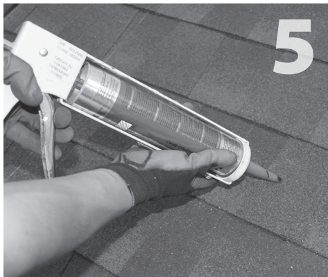
5 Clean off any sawdust, and fill hole with sealant compatible with roofing materials.
