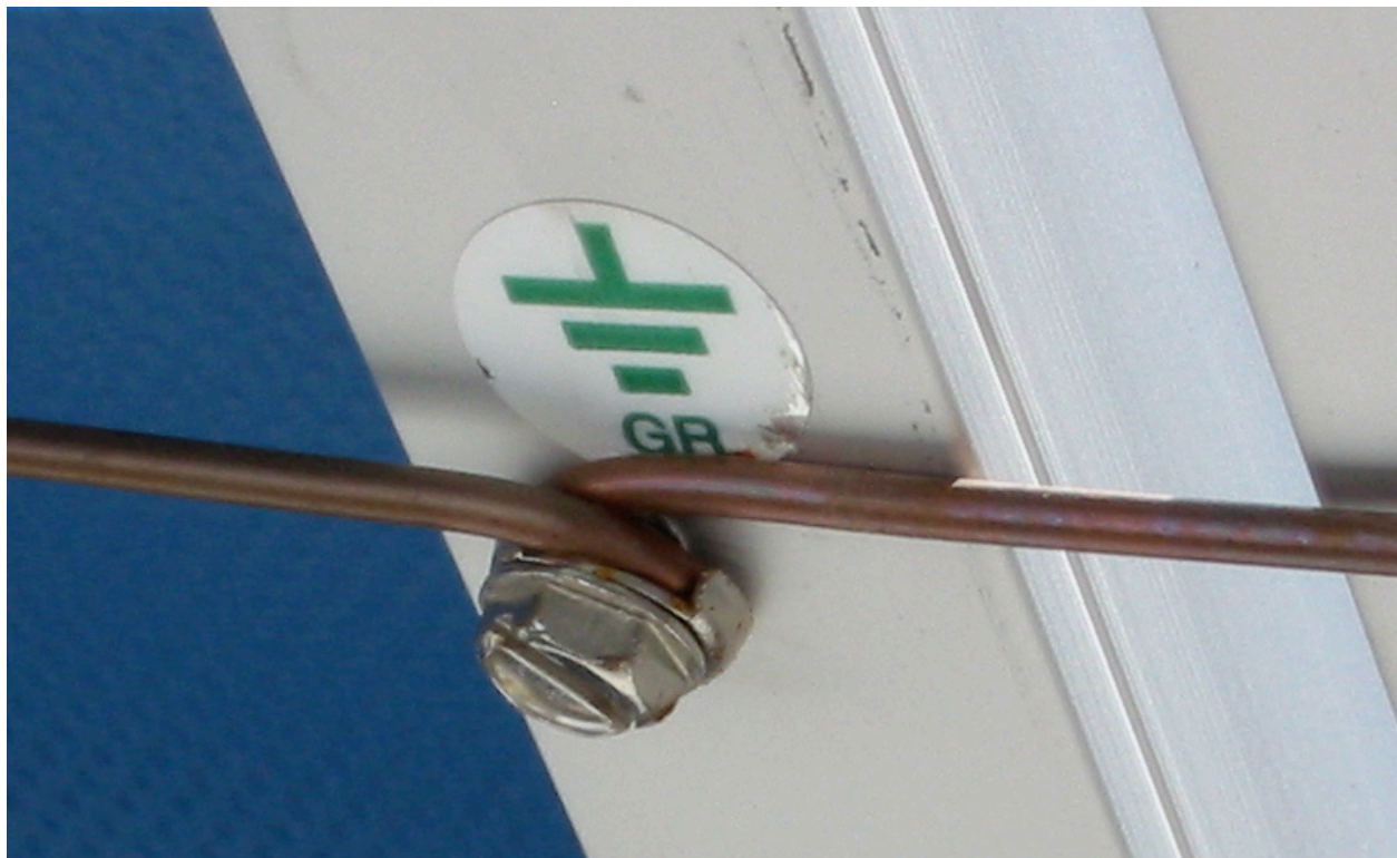
Figure G-3. Improper Module Grounding
